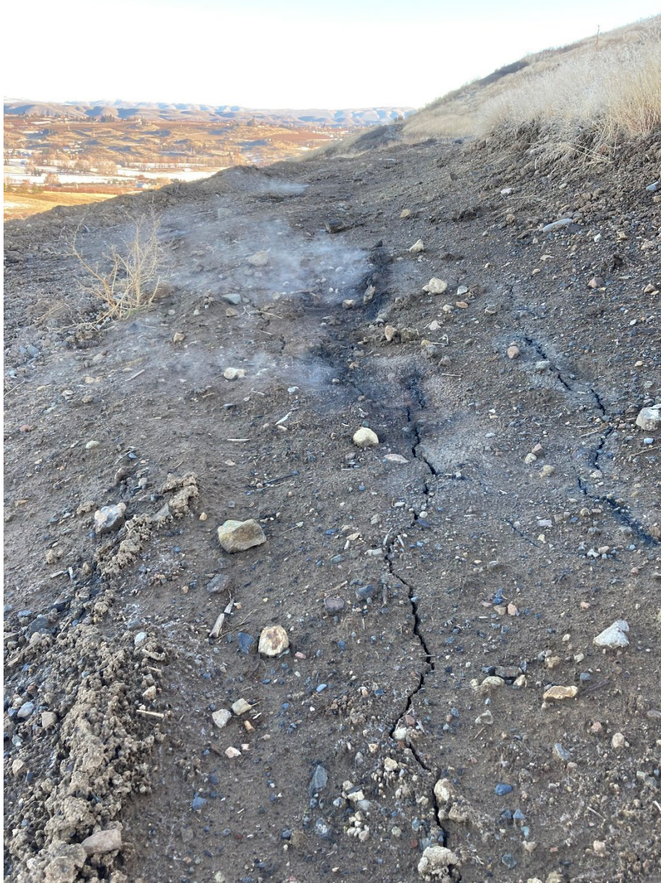
Figure 10: Facing north. Fine cracks in upper road above repaired slope with black residue around cracks and smoke/vapor emanating from cracks.
