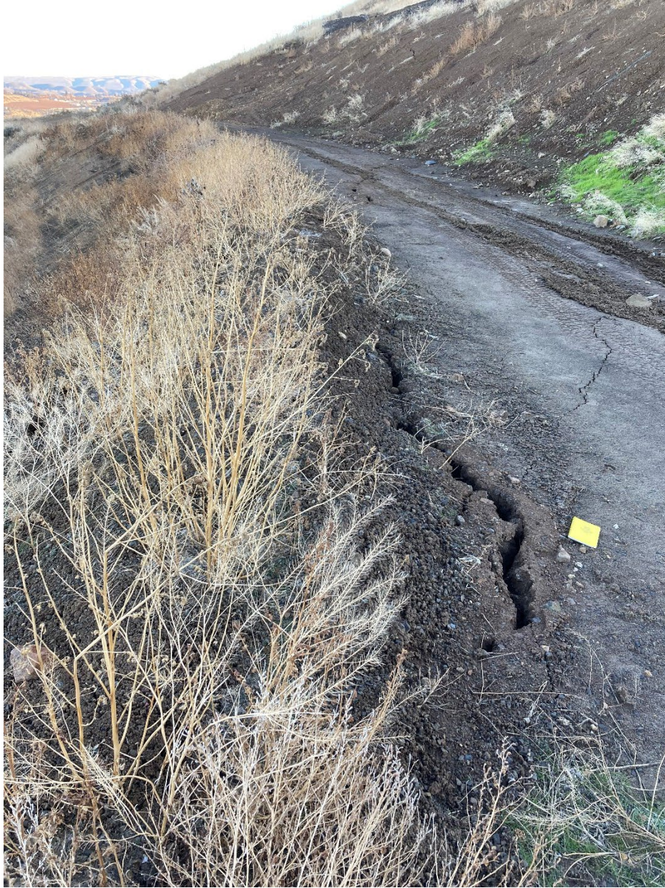
Figure 5: Cracks on perimeter landfill road. Note green vegetation on the opposite side of the road.
