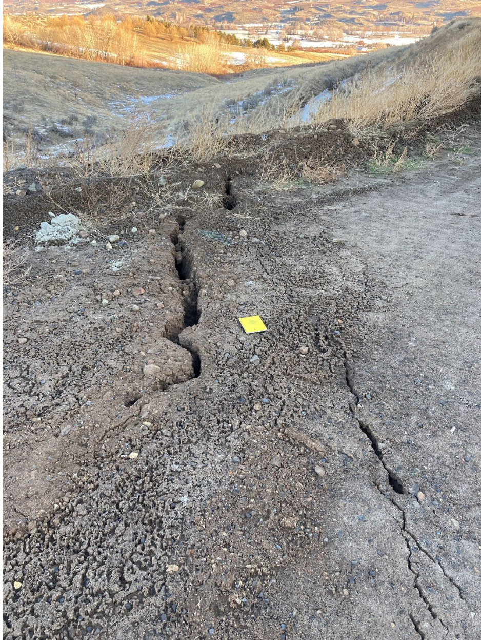
Figure 4: Cracks on perimeter landfill road.
