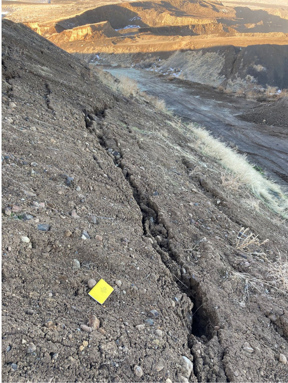
Figure 8: Cracks in slope above perimeter access road. Green vegetation directly below.
