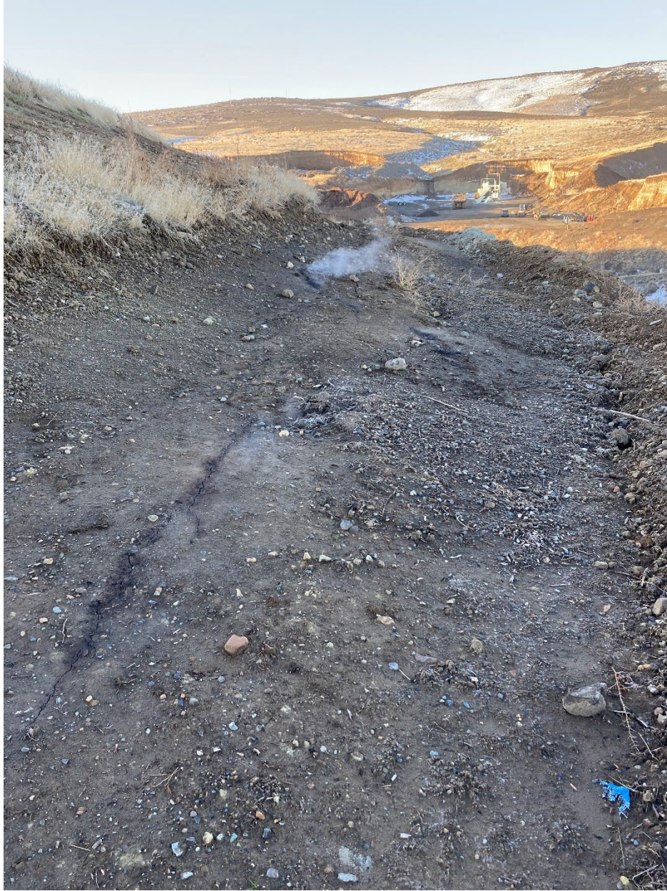
Figure 9: Facing south. Fine cracks in upper road above repaired slope with black residue around cracks and smoke/vapor emanating from cracks.
